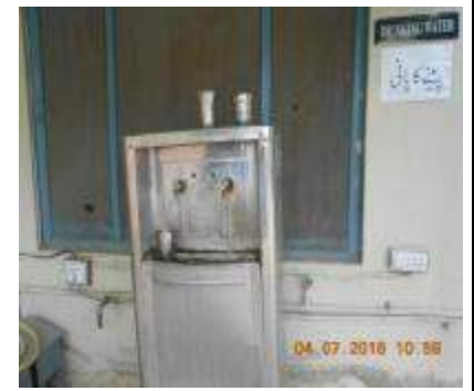
Drinking Water Point
